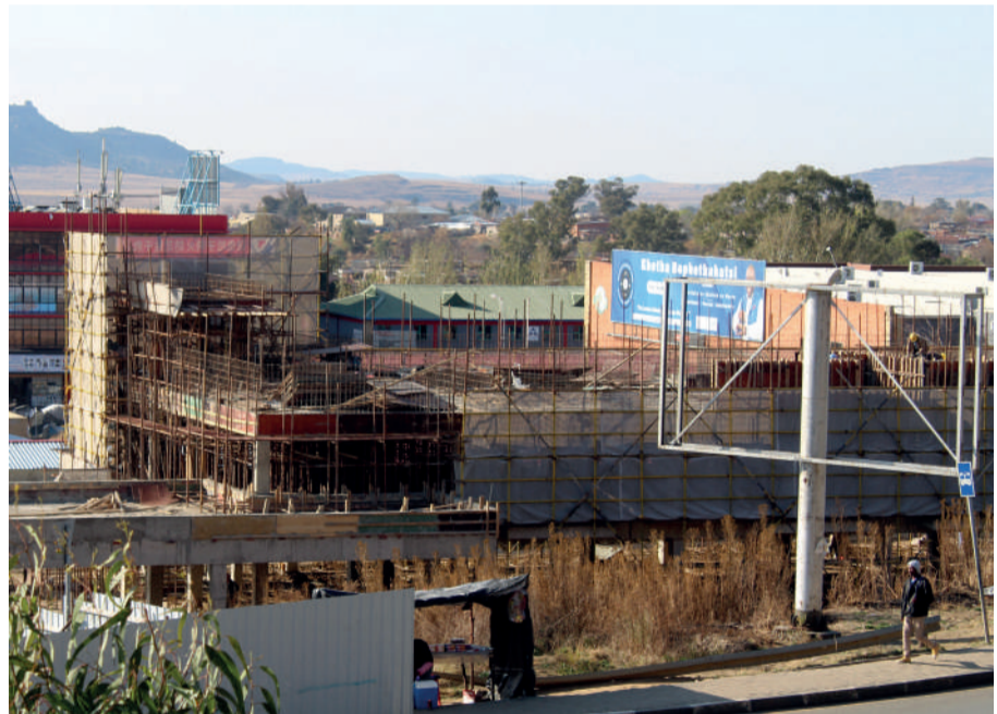
CONSTRUCTION of the Maseru District Hospital and Eye Clinic is ongoing at the disputed site.
