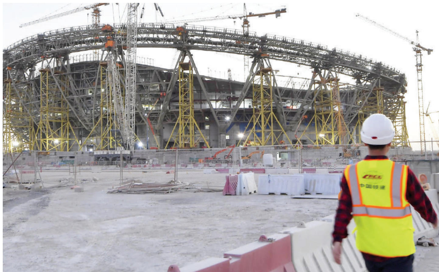
THE Lusail stadium, one of several new venues under construction for the 2022 World Cup in Qatar.
